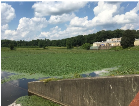
South Branch Pumping Station, August 2017
