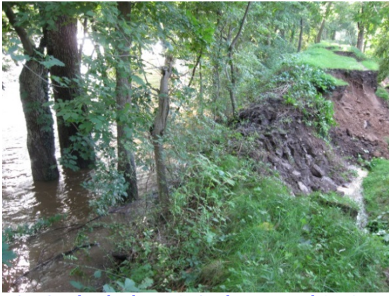
D&R Canal embankment in Stockton Borough in 2011.
