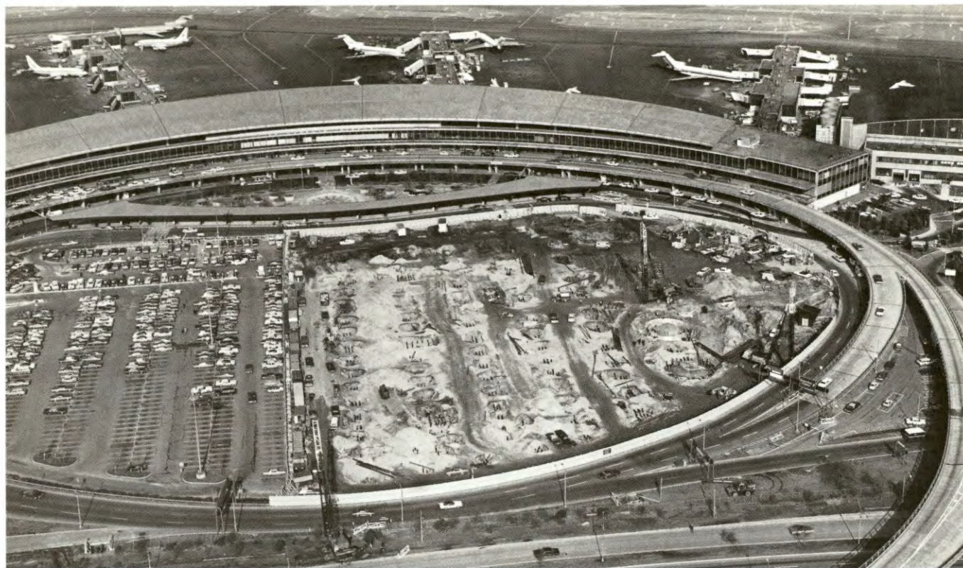
At LaGuardia Airport construction began in September on a five-level parking garage that will provide 3,000 additional parking spaces.
