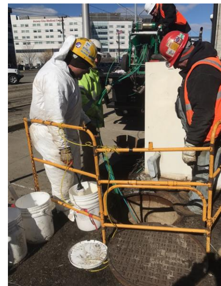
Hudson Bergen Light Rail Auxiliary Power Cable Pilot Program
