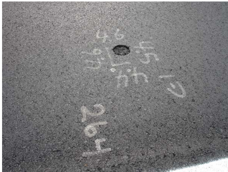
Figure 50 – Poor Backfilling of Extracted Core from Rt 202S in New Jersey
