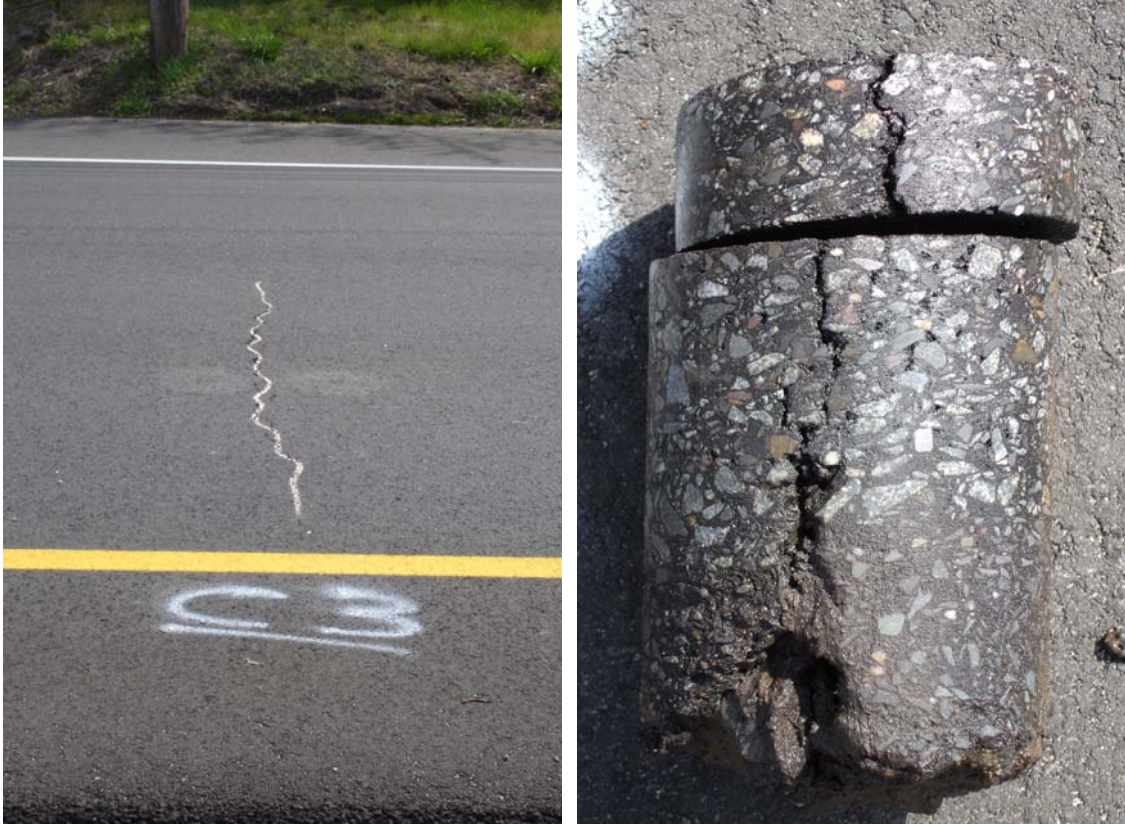
Figure 39 – Early Reflective Cracking in Test Section MP 2.5 to 4.5
