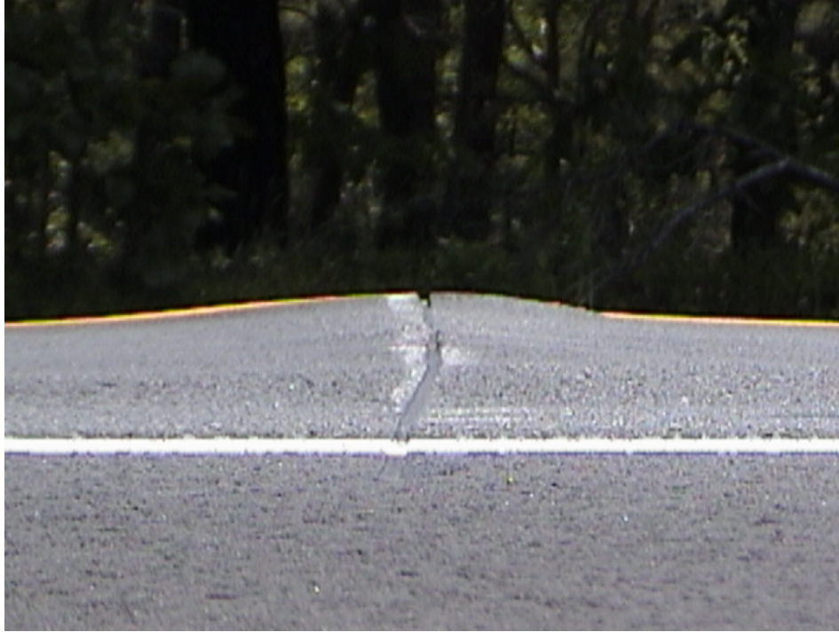
Figure 5 – HMA Overlay Failure at Joint Area Due to Excessive Curling Forces (Route 34 MP 11.5 Southbound)
