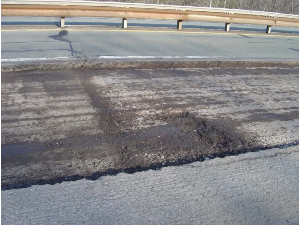
Figure 60 – Milled and Unmilled Surface of Interstate 476 in Pennsylvania
