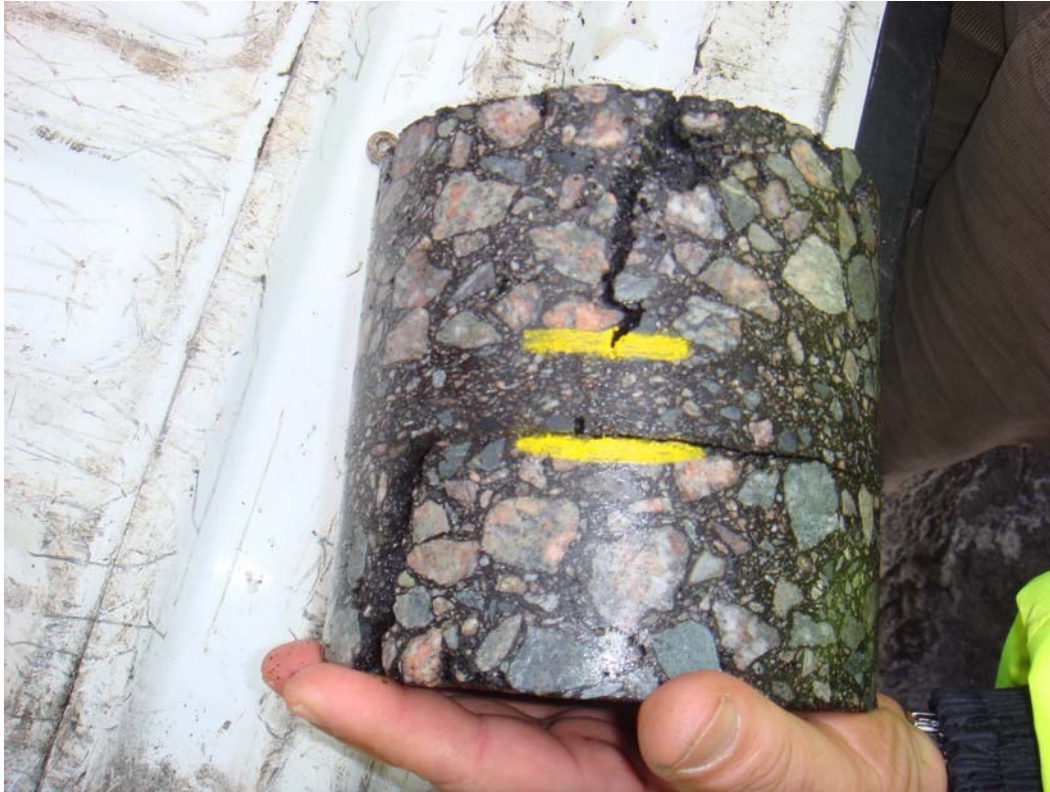
Figure 94 – Photo of Core Taken Through Surface Crack on I495 in Massachusetts
