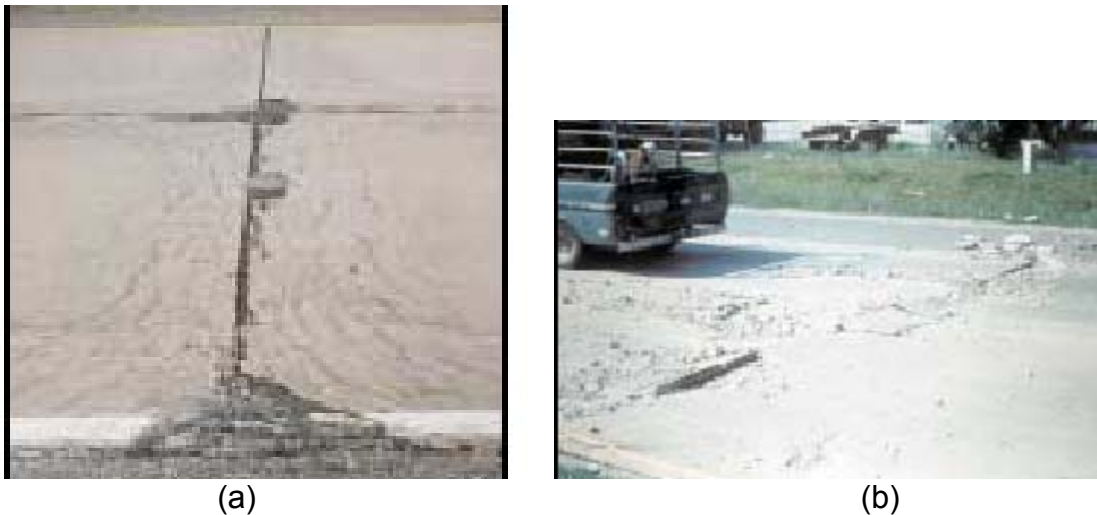
Figure 7 – (a) Durability Cracking (D-Cracking) of PCC Pavement; (b) Blow-up of PCC Pavement
