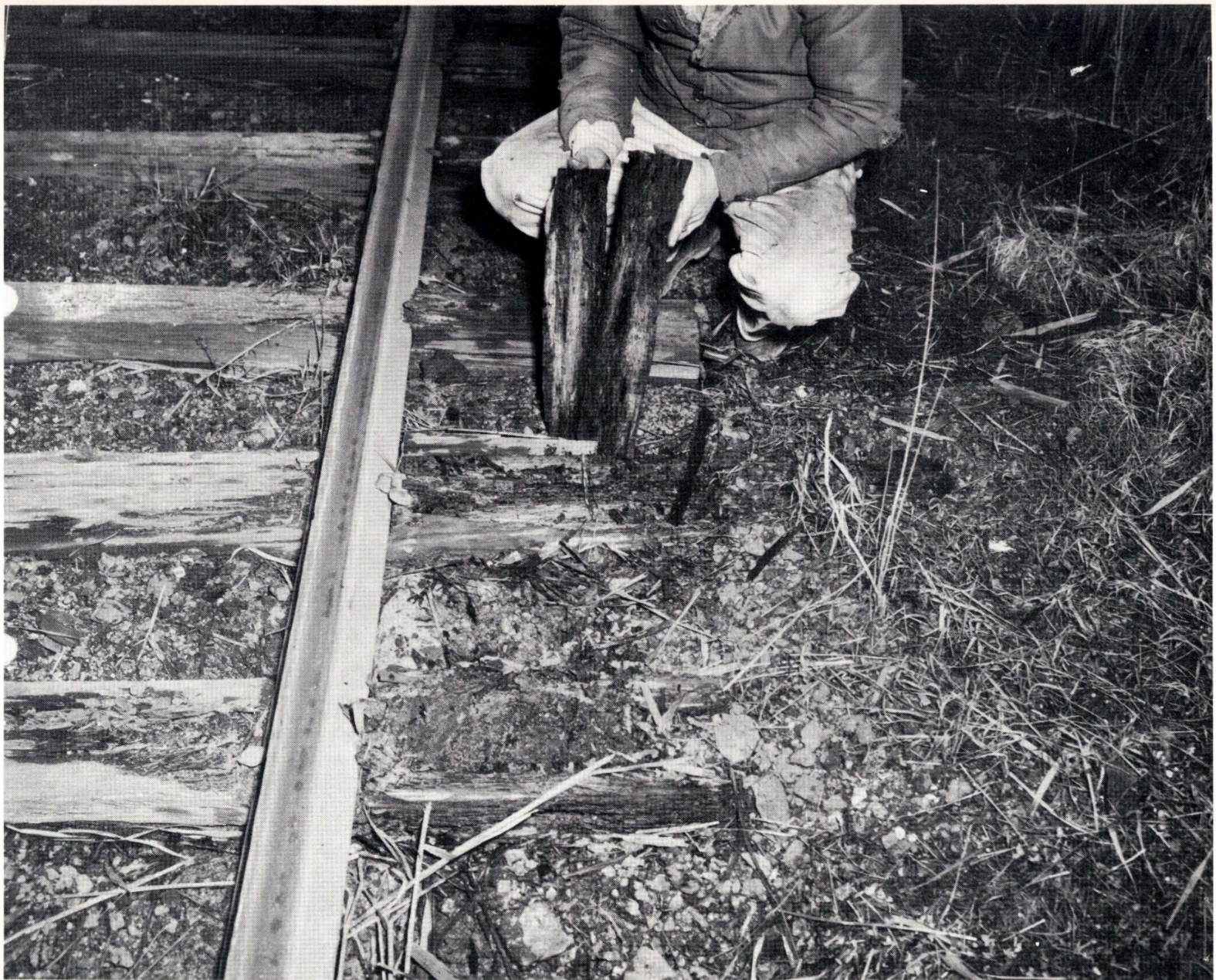
ROTTED TIES AND DETERIORATED ROADBEDS THROUGHOUT THE 22 MILES OF RAILROAD TRACK CHARACTERIZED THE SEAPORT WHEN PORT AUTHORITY ASSUMED RESPONSIBILITY IN 1948.
