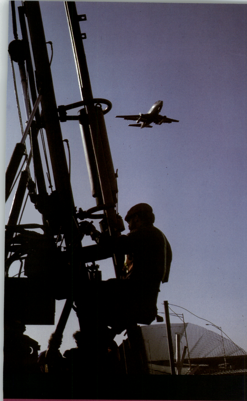
DRAMATIC silhouette of equipment operator replacing guardrail posts on dual/dual mainline where Turnpike skirts Newark International Airport.
