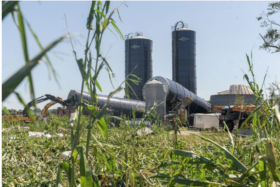
Figure 20: Tornado Damage at Wellcrest Farms in Mullica Hill, NJ, September 2, 2021@
