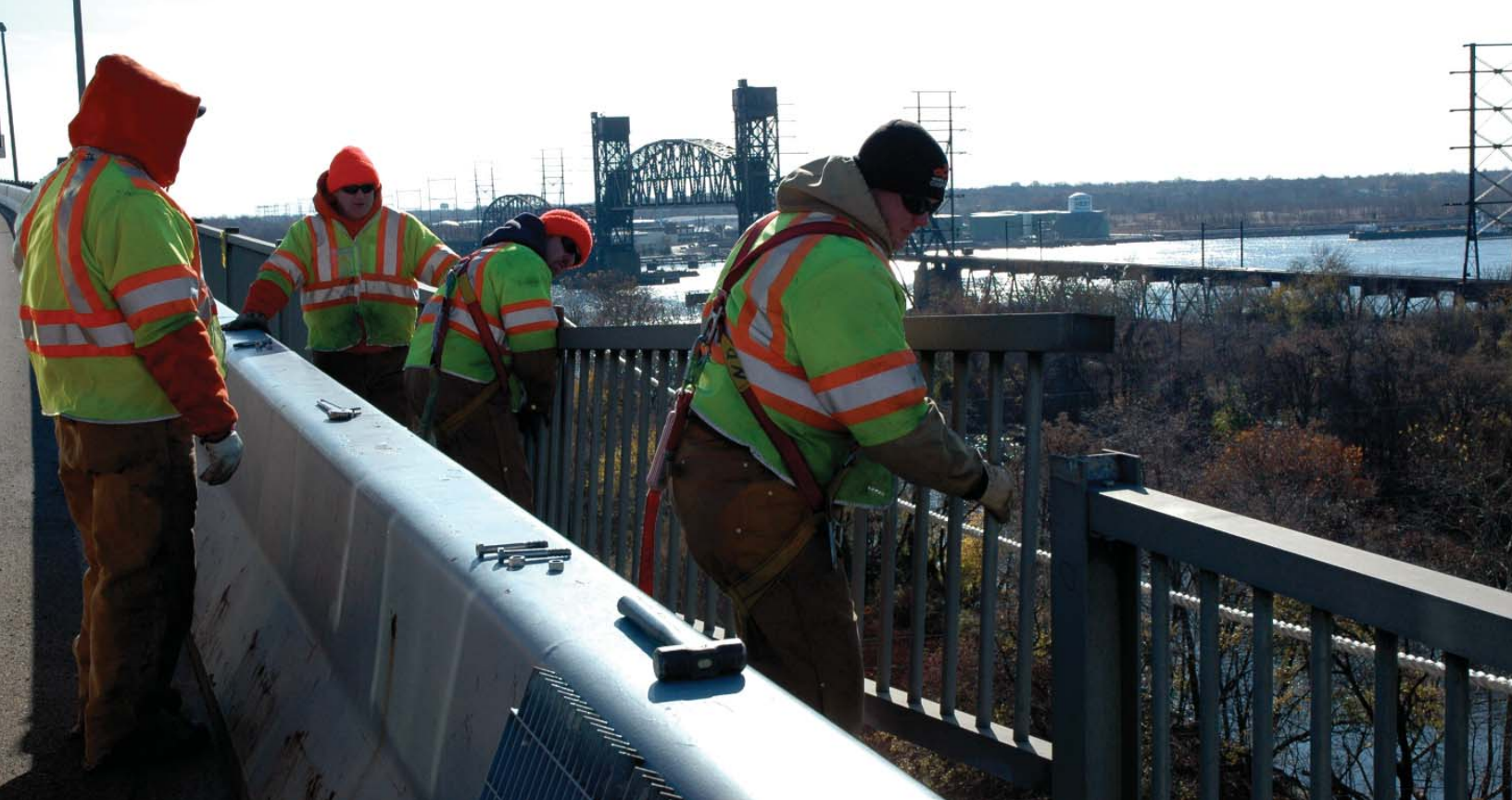
▲ Betsy Ross Bridge – Construction and Maintenance workers replace anchor bolts that hold the handrails in place.
