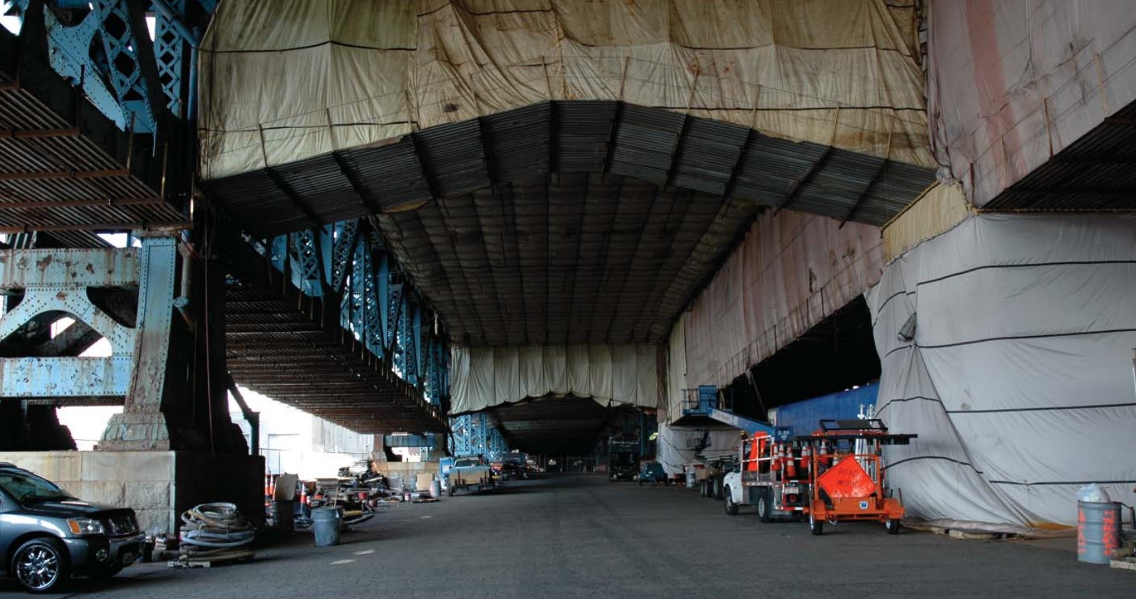
▲ BFB Painting Project – View of the containment area under the Ben Fran lin Bridge in Philadelphia. The containment provides a shield that protects the environment from particles removed as a result of blast cleaning. Total project cost is $87 million.
