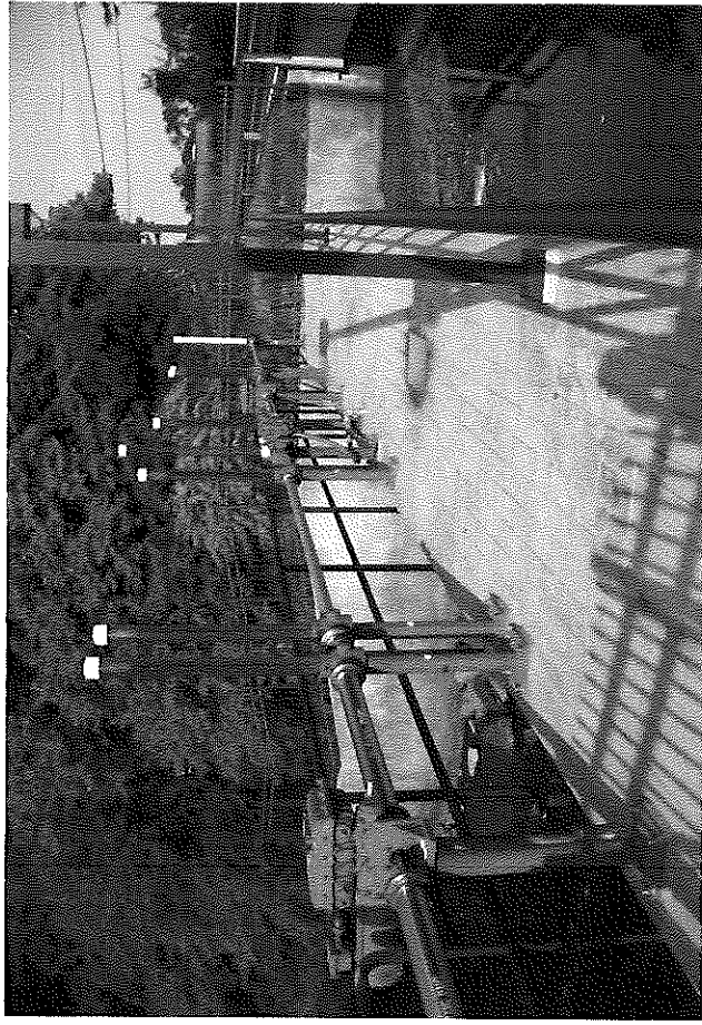
Kirby's Mill motors on walkway
