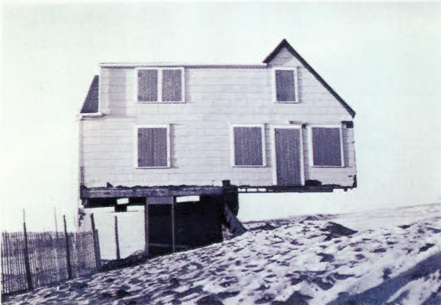
Severely eroded sand left this house at Barnegat Light standing precariously on its pilings.
