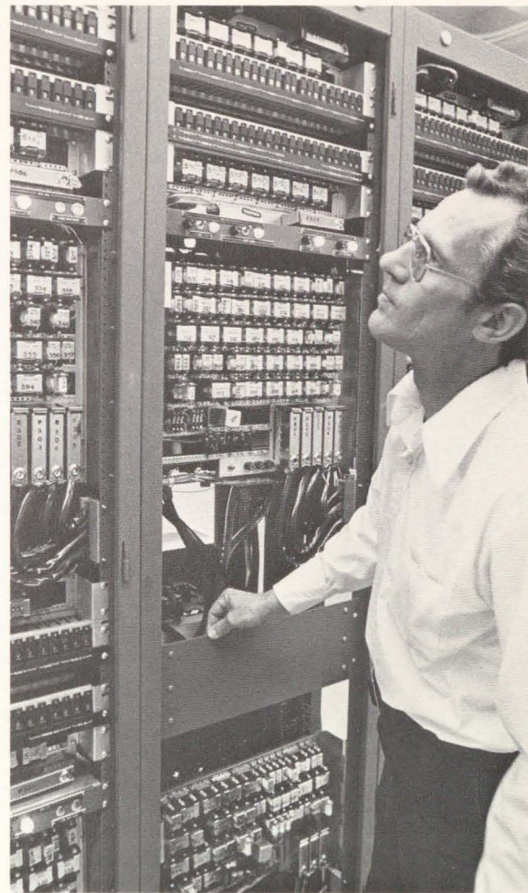
Electronics technician checks toll monitoring equipment.
