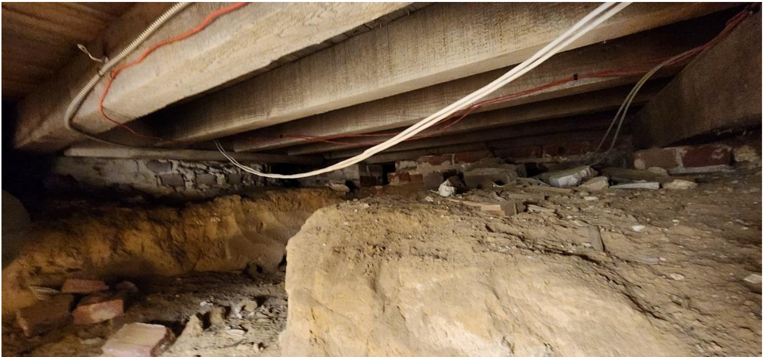
View of the crawlspace looking northeast showing how portions of the crawlspace have been dug out.
