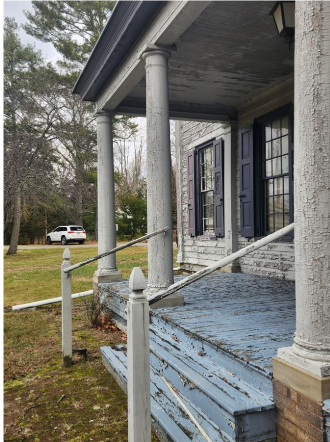
View of the front porch showing wholesale paint loss, which is throughout the painted porch elements.
