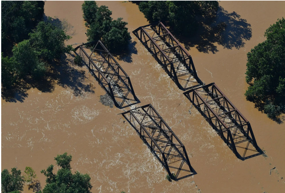
Figure 15 : Bridge in Somerset County Inundated by Floodwaters
