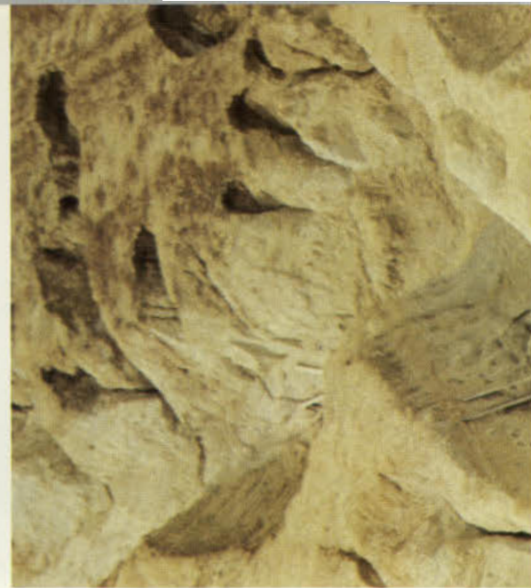
Eroded gullies—some up to 40 feet deep, resulted after this development site was stripped of its natural vegetative cover and later abandoned.
