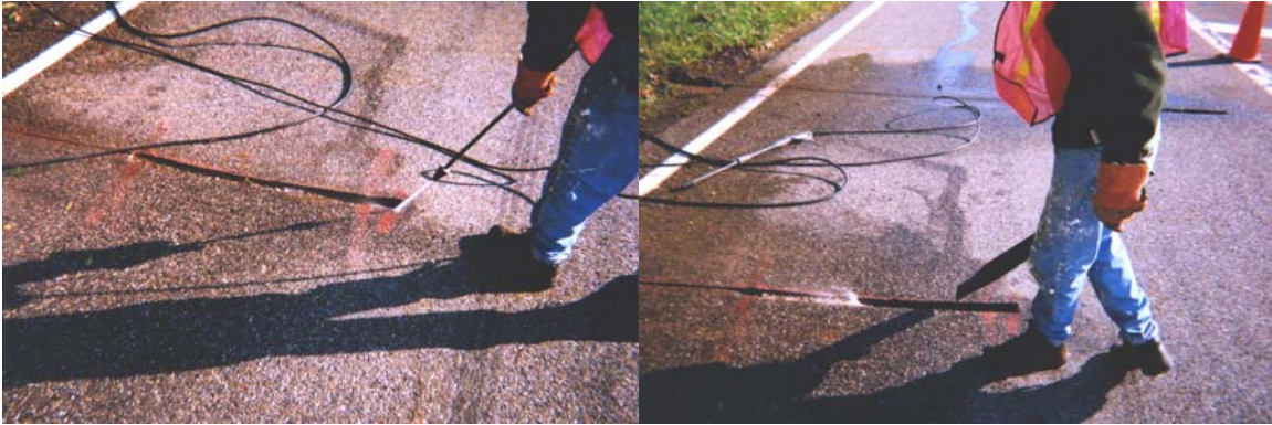
Figure 59 Photograph showing the power washing and blowing of the groove to remove debris and water.
