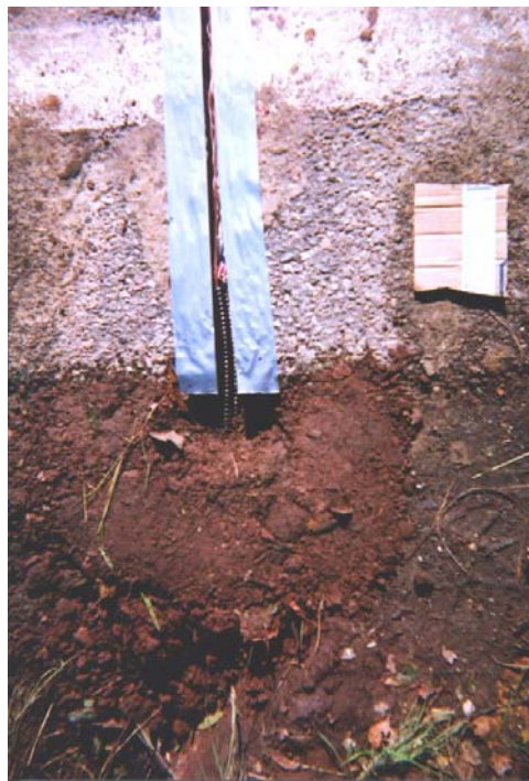
Figure 60 Photograph of the groove with the wires and plastic conduit ready for epoxy infiltration.
