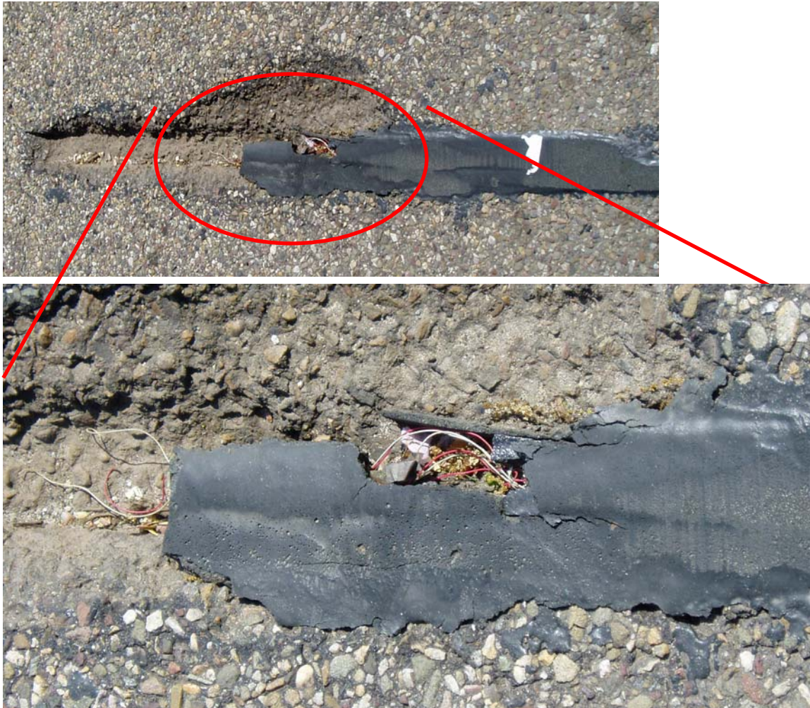
Figure 77 Close-up examination of failed outside of lane sensor assembly.
