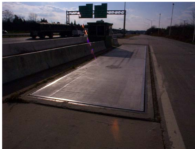
Figure 49 Route 287 weigh station static scale.
