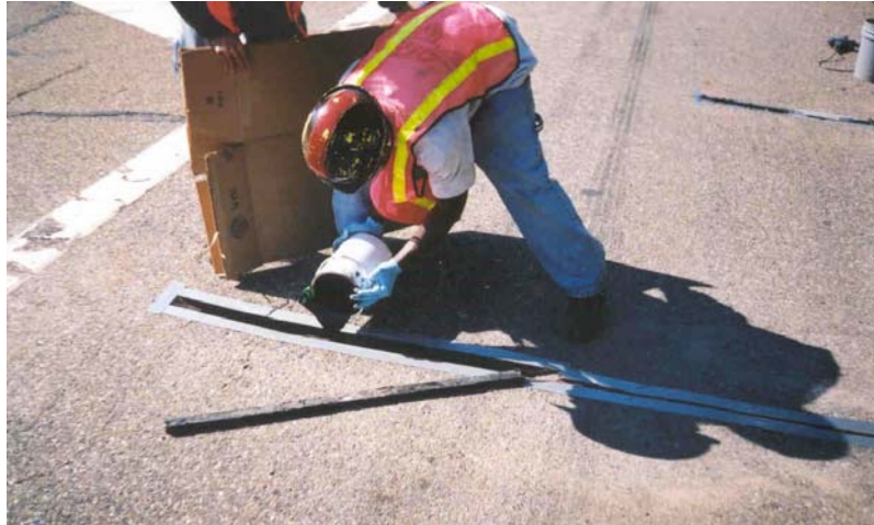
Figure 62 Photograph of PU-200 epoxy being placed in the bottom of the groove prior to final placement of the sensor assembly.
