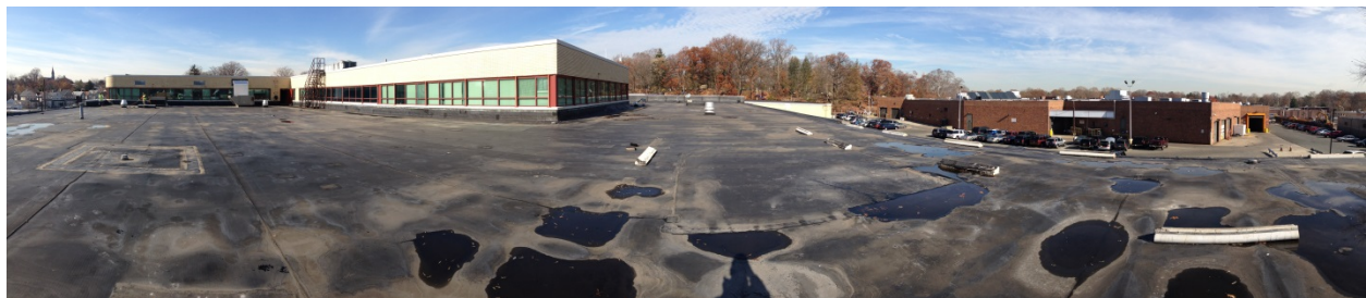
Orange Annex - Roof Damage
