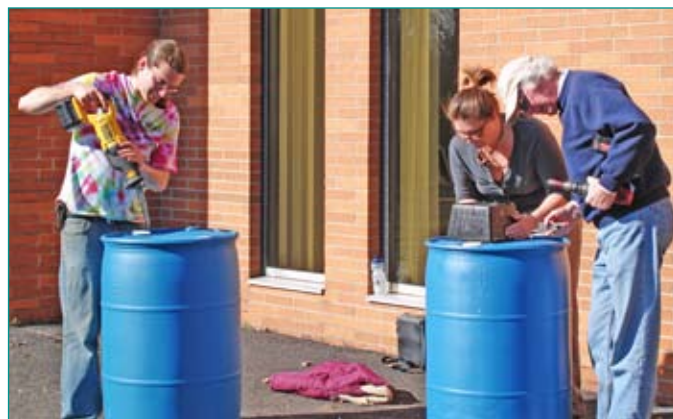
Rain barrels under construction at the March 2010 workshop held behind the DRBC building in West Trenton.
