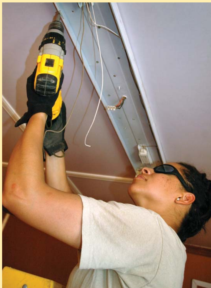
Staff Sgt. Anne McKenzie, Electrician, installs an overhead light fixture in the new Gryphon Air facility.
