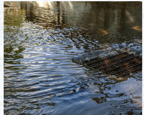
Pluvial flooding overwhelming stormwater systems
