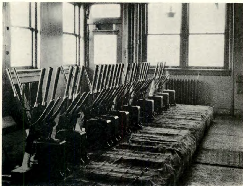
Interlocking Signal Station on Belt Line No. 13, with interior view showing battery of switch levers.
