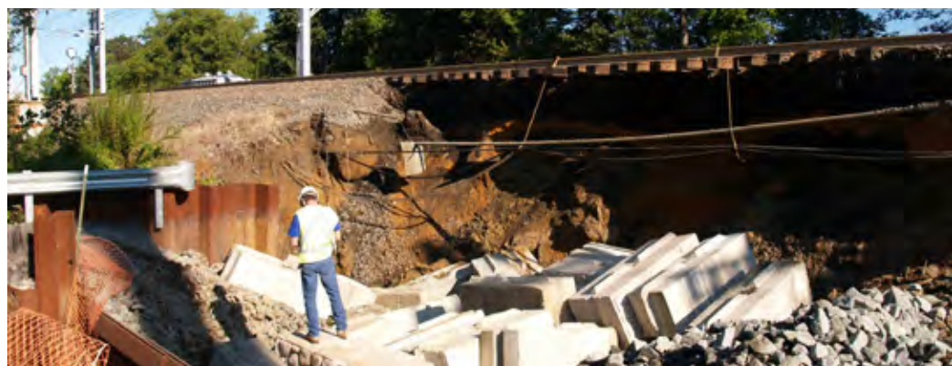
Large portions of railroad beds were washed out during Hurricane Irene.
