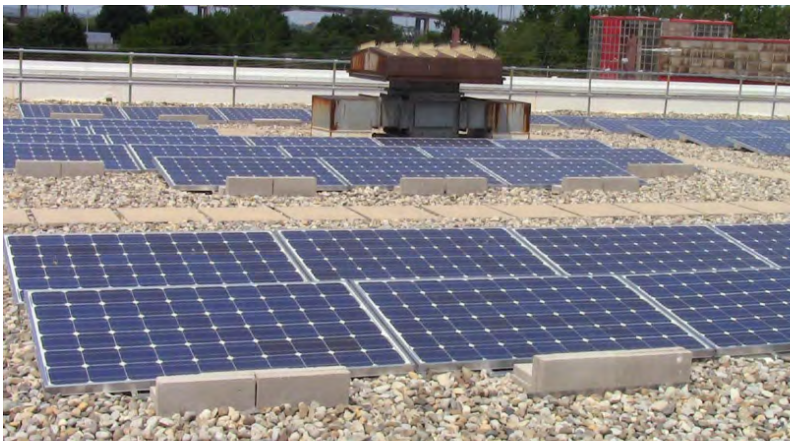
Solar power has been installed at the Meadows Maintenance Complex, our largest rail maintenance facility.
