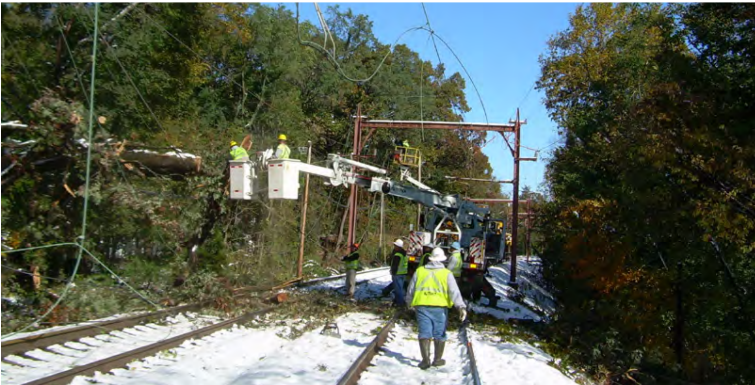
A freak snowstorm in October 2011 caused extensive damage to more than 50 miles of railroad infrastructure, particularly on the Morris & Essex Lines.
