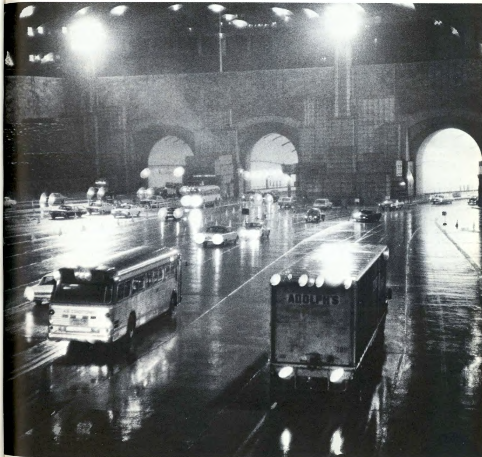
The repaving of the north tube of the Lincoln Tunnel, the world's only three tube underwater crossing, and portions of the New York and New Jersey Plazas was completed during the Fall.
