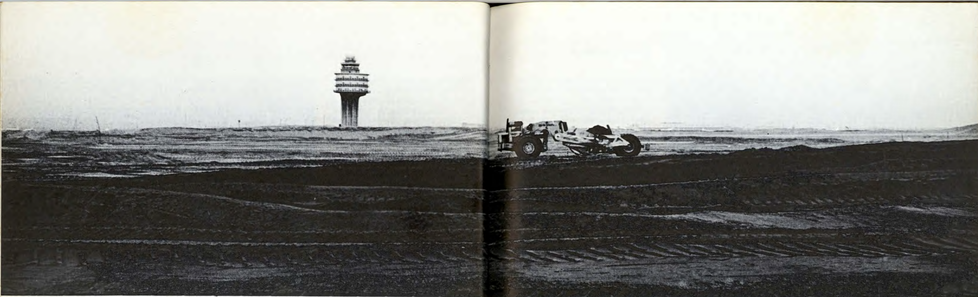
With some sections reaching a height of twenty-five feet, more than 14,000,000 cubic yards of hydraulic fill have been placed on a 450-acre area to prepare
