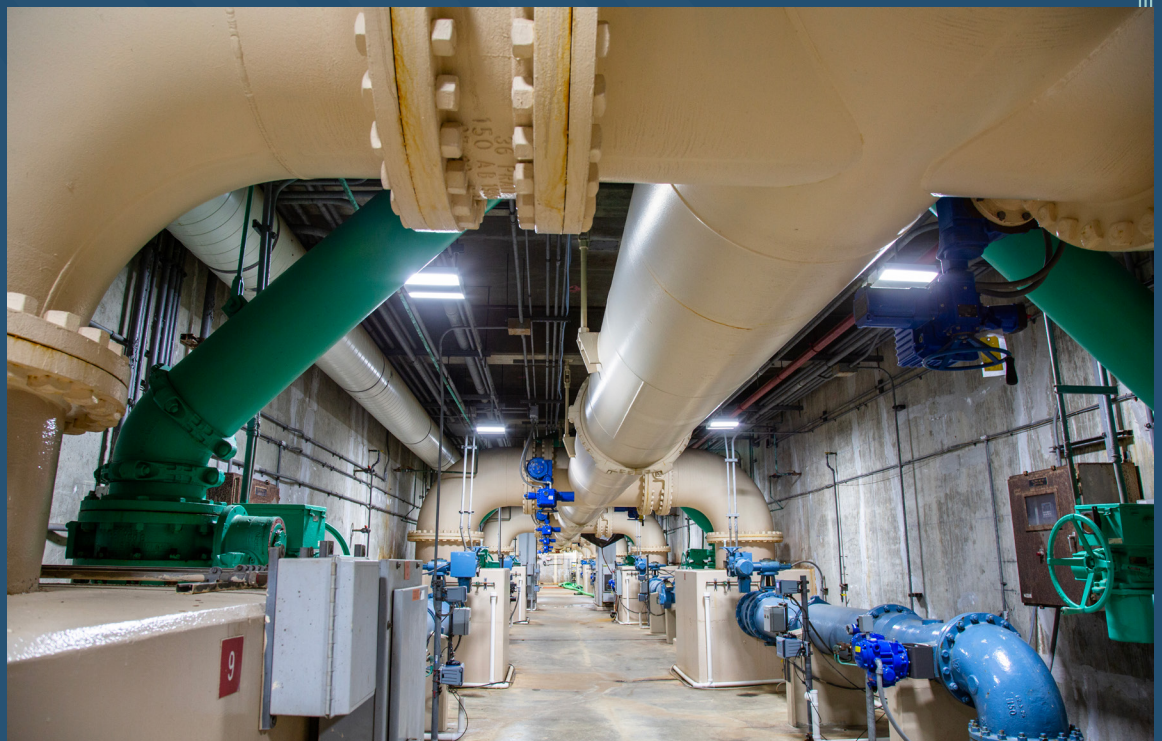
Water treatment in Veolia's Haworth Water Treatment Plant in Haworth.
