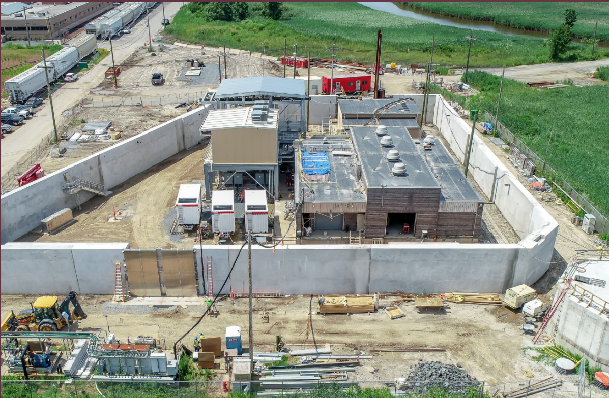
Middlesex County Utilities Authority's Sayreville Pump Station with a flood wall constructed around the facility.
