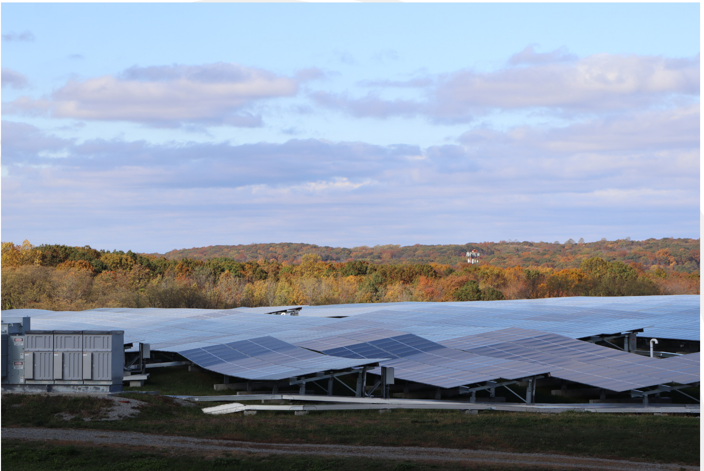
Solar panels installed at Combe Fill North Landfill in Mount Olive.
