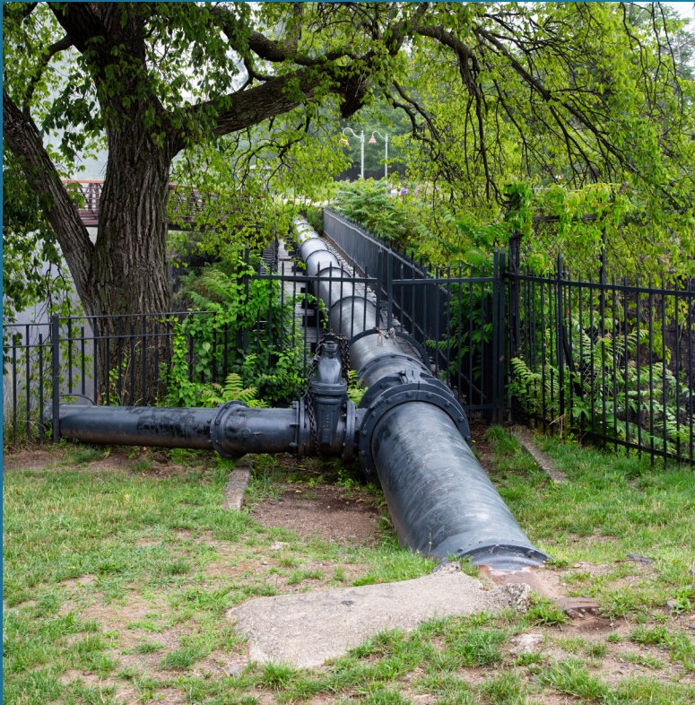
A water pipeline located in the Paterson Great Falls National Historic Park in Paterson.
