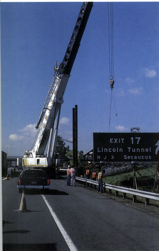
NEW SIGN bridge was constructed in Secaucus to hold variable message and exit signs. Here Exit 17 is hoisted into place.
