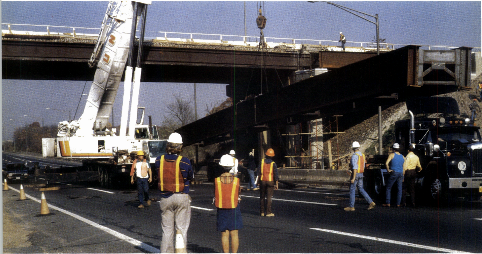
PLACING GIRDERS in Interchange 9 northbound ramp construction as part of the 1985-90 Widening Program. Each set weighs 50 tons and is 90 feet long.
