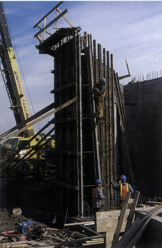
BRIDGE PIER is in place to hold fly-over ramp for southbound inner roadway traffic from Interchange 9.
