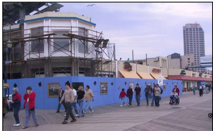
Right: Siganos Boardwalk Properties, Inc. continues work on the $2 million makeover of the 1700 block of the Atlantic City Boardwalk. Siganos Plaza is scheduled to open in May 2003.
