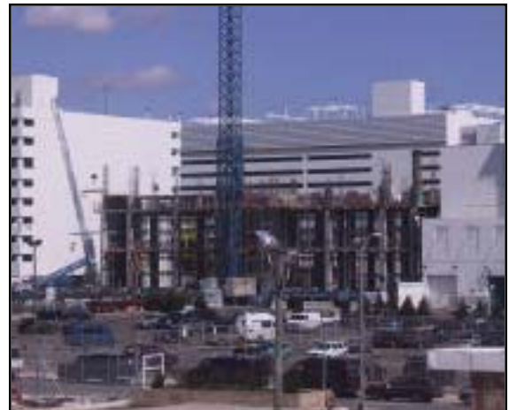
Construction of Resorts 459-room hotel tower is underway. The tower should be completed by spring 2004.
