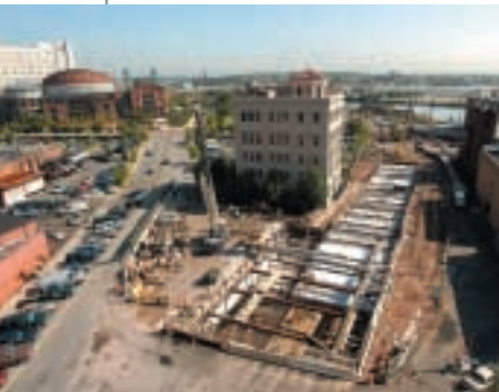
The extension of the Newark City Subway to Newark Broad Street Station will improve connectivity in downtown Newark.
