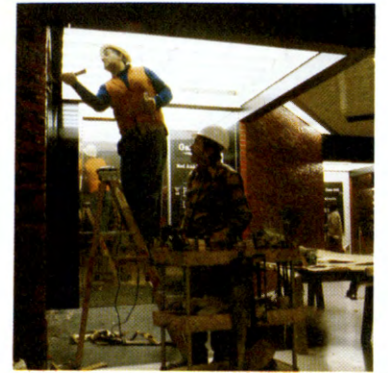
At work on the modernization of the Port Authority's midtown bus terminal.
