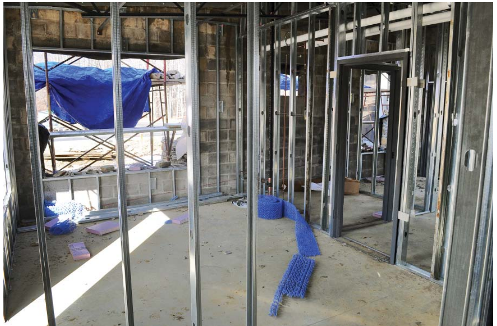
The Public Information Center office wall structure is defined with the addition of studs, sill plates and door openings. (New Jersey Department of Military and Veterans Affairs photos by Kryn P. Westhoven/Released)
