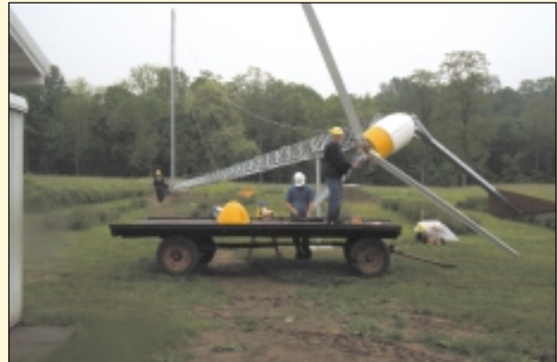
This wind turbine was recently installed on a preserved farm in Burlington County, New Jersey.
