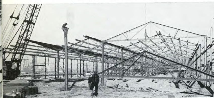
Erection of steel framework at Pier 11, Brooklyn-Port Authority Piers, was major step toward completion of the terminal.
