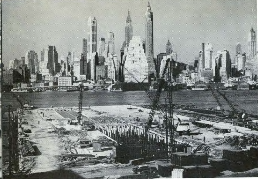
Construction of $5,100,000 Pier 2 of the Brooklyn-Port Authority Piers, was 45 per cent complete by the end of 1957.
