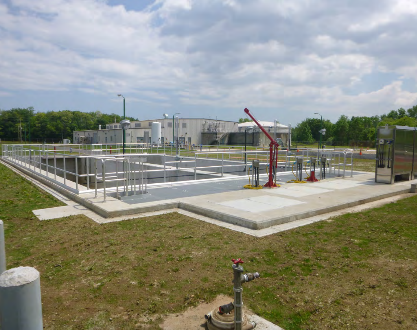
Southeast Monmouth MUA | Manasquan Water Treatment Plant Equalization Basin SFY2013 Loan: $8,821,000
