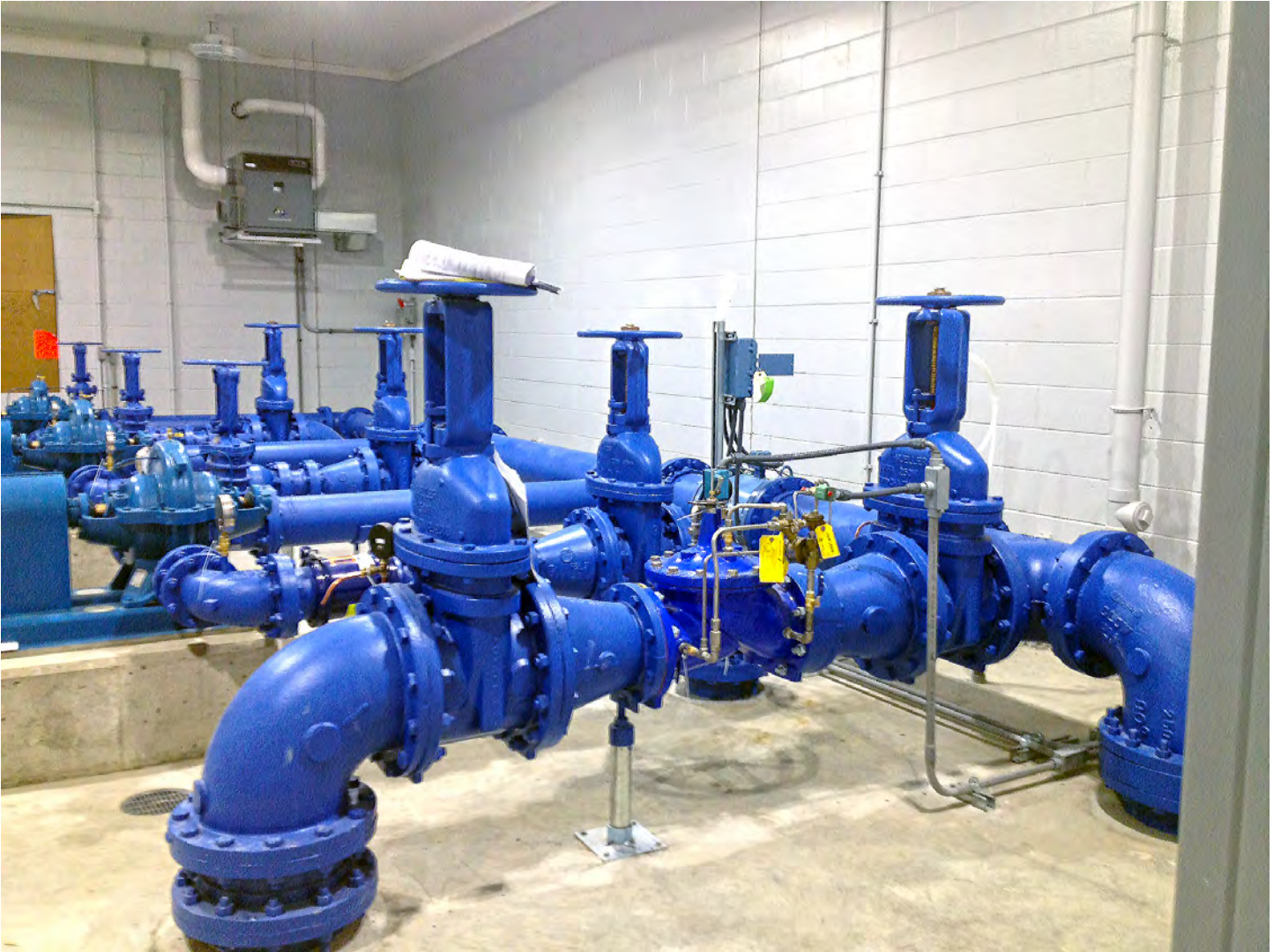
Millville City | Geissinger Well No. 18 Booster Pumping Facility SFY2013 Loan: $2,885,775
