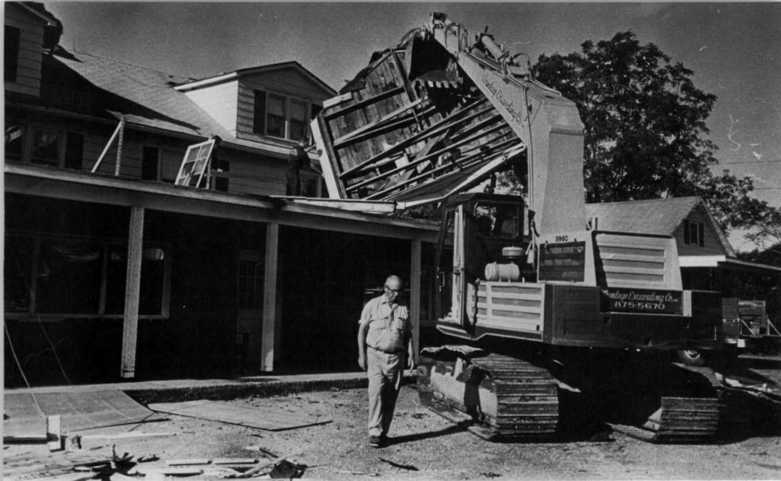
Owner Ralph Space looks on as workmen remove a section of roof 50 feet from its original position (Tornado date: Sept. 2, 1980)
