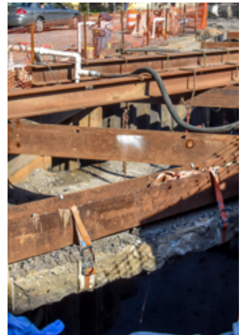
Camden County MUA, Wastewater Treatment Plant Improvements. SFY2021 Loan: $8,056,643
