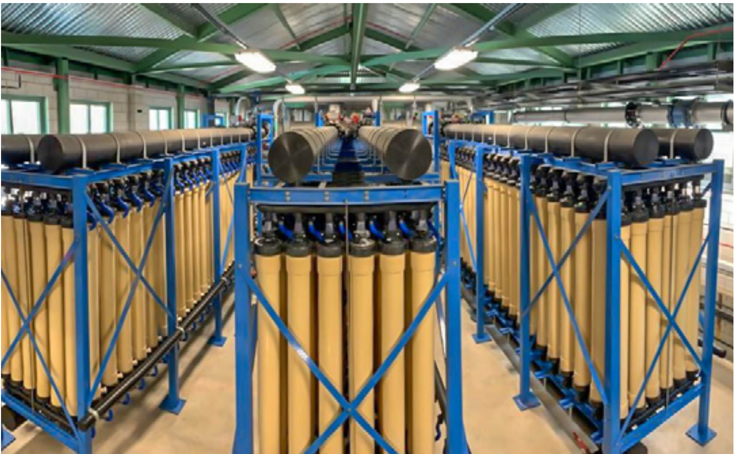
North Bergen MUA Woodcliff Wastewater Treatment Facility Improvements. SFY2021 Loan: $19,725,440
