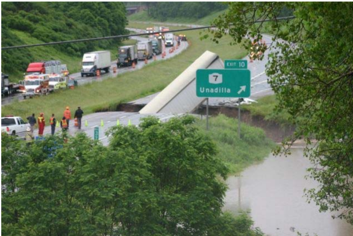
Figure 1. Collapse of New York State Thruway (I-88) due to culvert failure on June 28, 2006 (New York State Police Photo)
