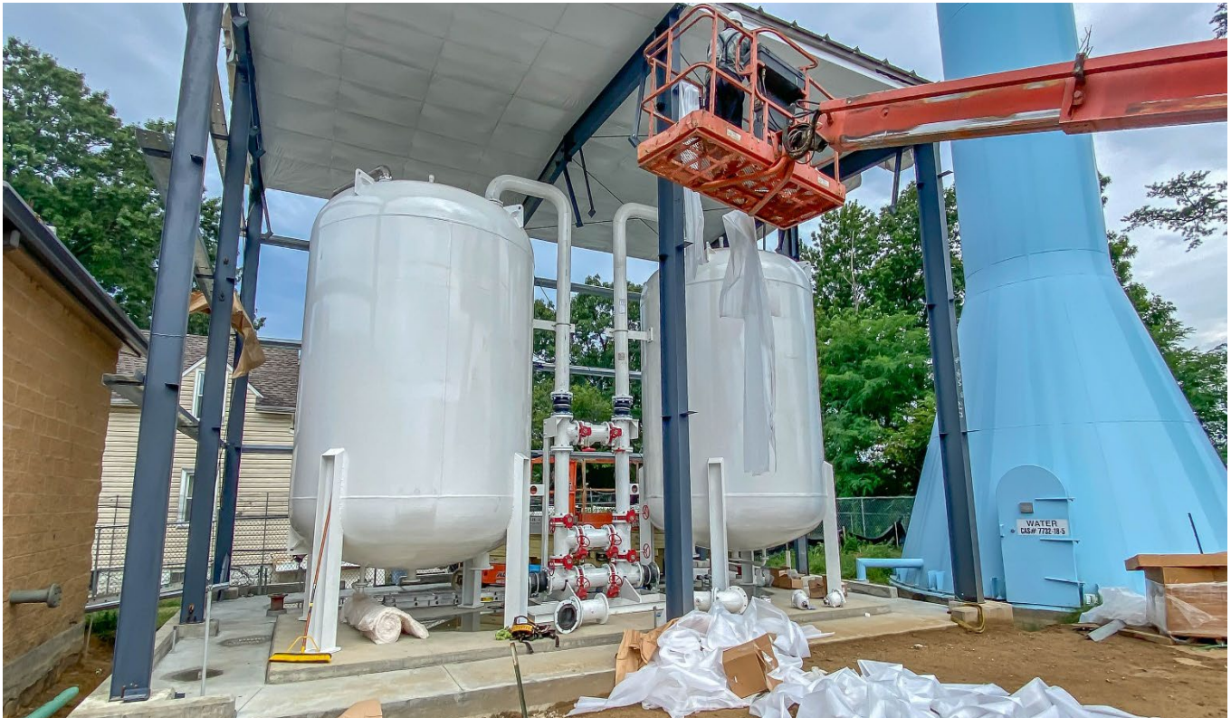
National Park Borough Addition of PFOS Treatment at existing water plant. SFY2024 Financing Program.
