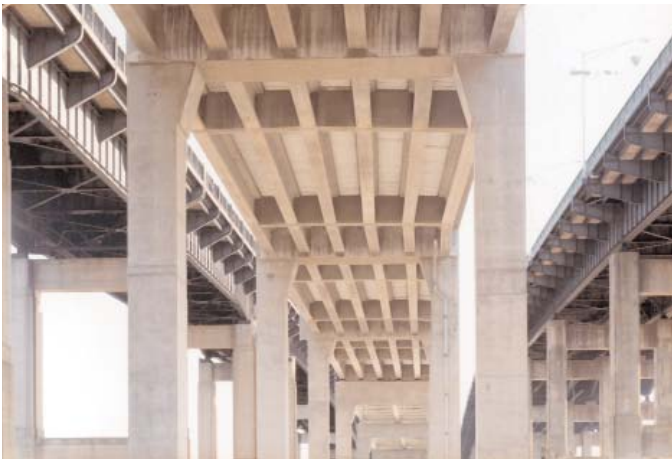
Garden State Parkway and Route 9 Bridges after Widening of Route 9 Note lower profile (top), pier changes (middle), and framing (bottom).
