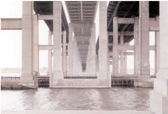
Garden State Parkway and Route 9 Bridges after Widening of Route 9. Note imitation of granite masonry at pier base (bottom).
