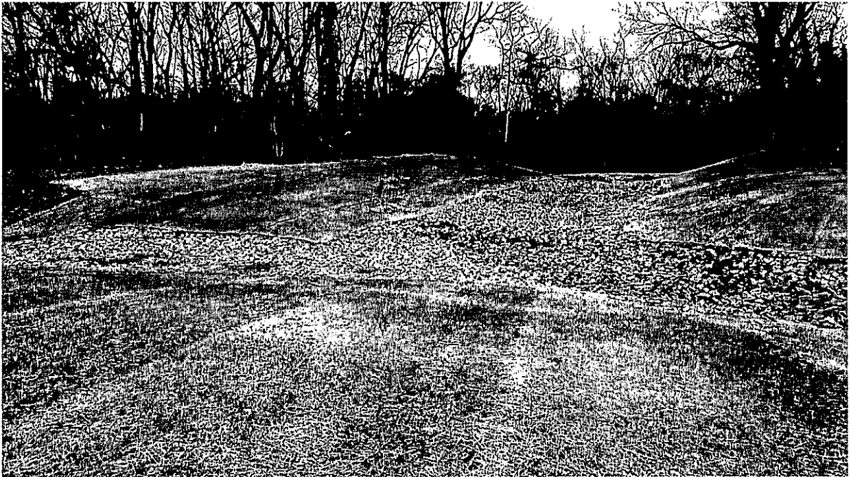
Figure 32: AFTER – check dams and grass mats after restoration to slow runoff into Barrett's Run. April 2019
