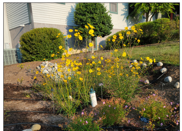
Above Top: Contractors installed bioretention soil at the site of the Commission's rain garden.
