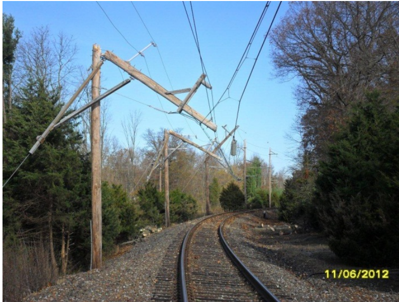
Wooden Pole Damage After Superstorm Sandy
