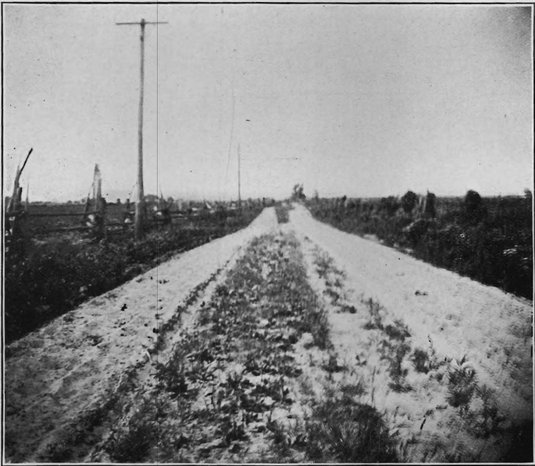
Pedricktown road, Salem Co., before improvement.
