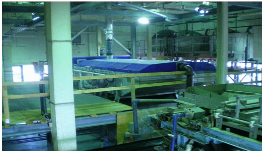
NEWLY INSTALLED BELT FILTER PRESS
