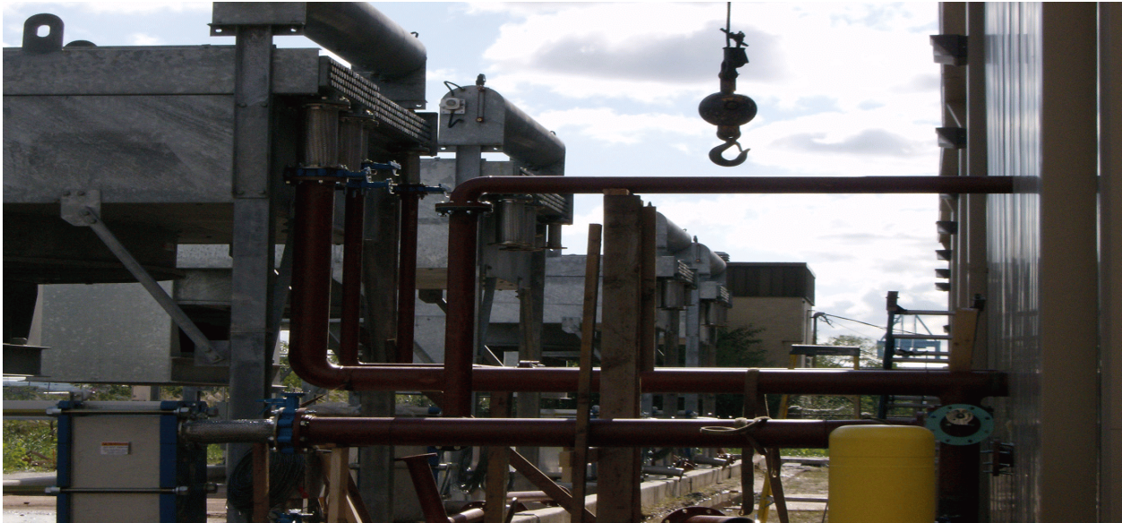
CO-GENERATION COOLING SYSTEM Photo Courtesy of Joint Meeting
