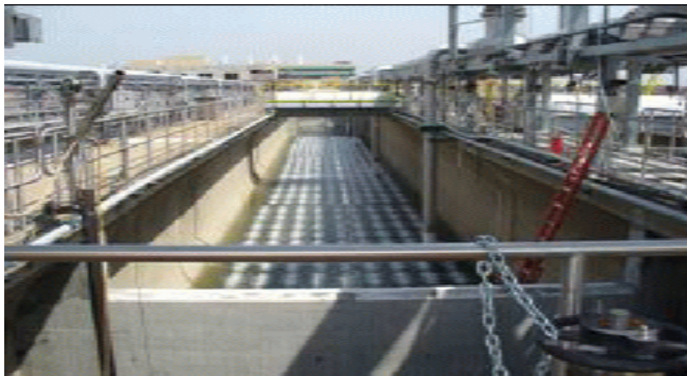
RETROFIT STEP FEED BNR Photo Courtesy of NYC DEP
