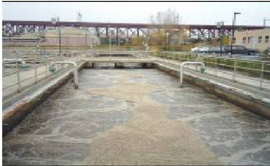
RETROFIT STEP FEED BNR Photo Courtesy of NYC DEP
