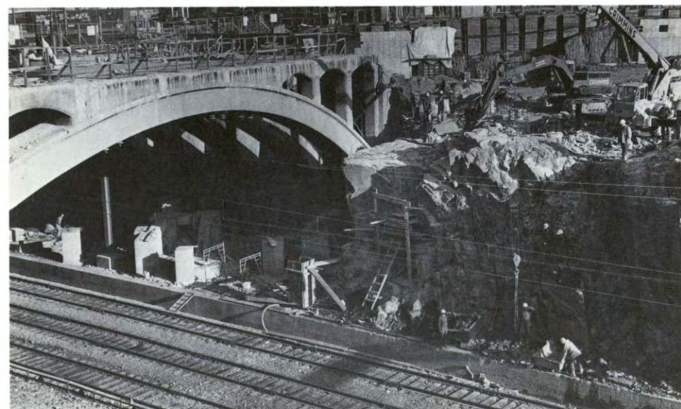
The Journal Square platforms are being extended to accommodate longer PATH trains.
