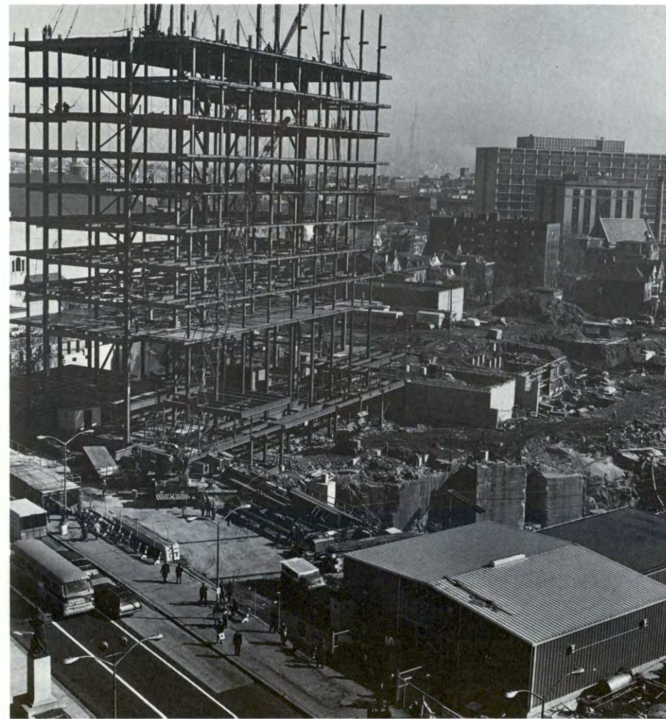
Structural steel rising for the ten-story PATH Administration Building, part of the coordinated Journal Square Transportation Center in Jersey City. At lower right is PATH's new temporary Journal Square station entrance.
