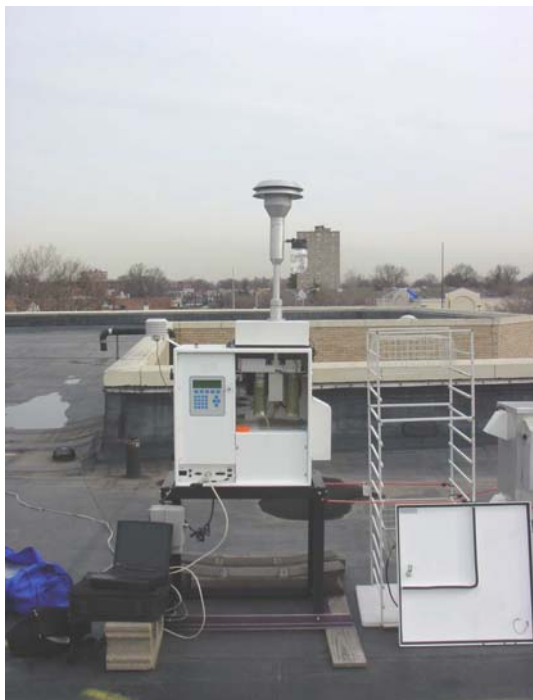
USEPA-approved manual PM 2.5 sampler on the roof of the Mitchell Building in downtown Elizabeth
