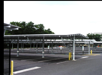
Above: Solar panel carports were installed above the parking lots at Stockton University in Galloway Township.
