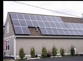
Above: Solar panels in Pemberton Township.
