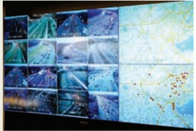
Traffic Management Center (TMC) video screen display
