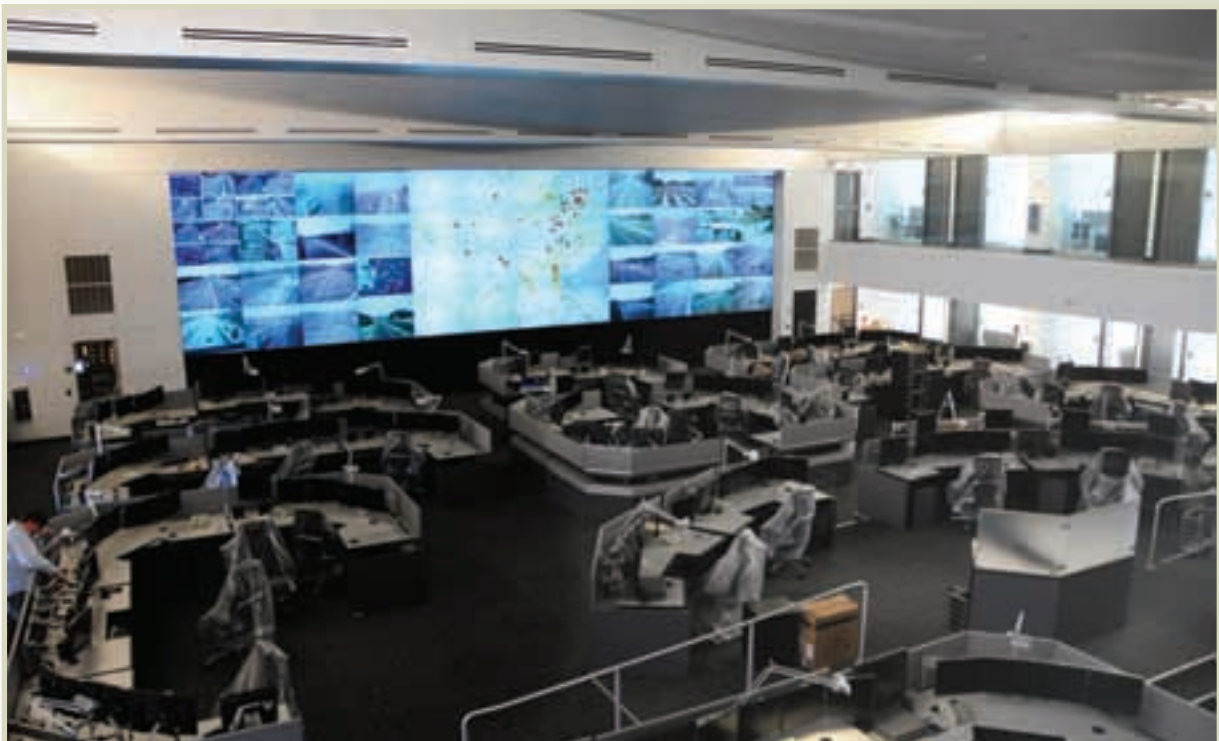
Inside the Traffic Management Center (TMC)
