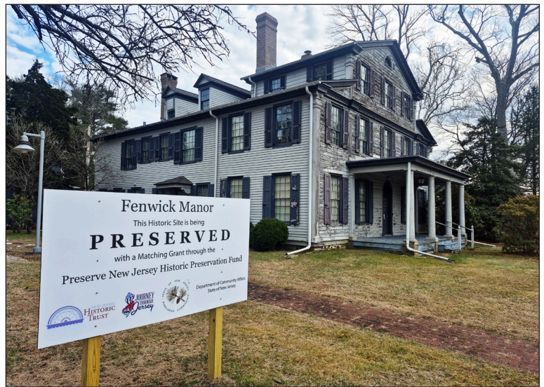
Above: In 2025, the Commission took significant strides toward rehabilitating one of its principal office buildings, Fenwick Manor.
