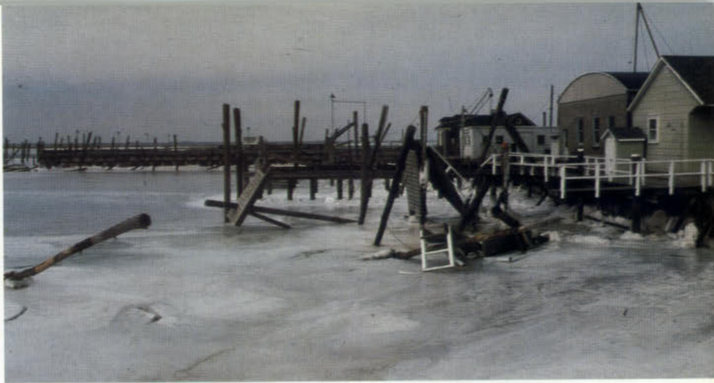
Man-made structures were severely damaged by the extreme cold. Ice action has lifted pilings and tilted docks in this photo.
