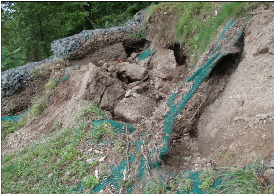
Loss of the embankment along the RiverLINE – Hurricane Irene
