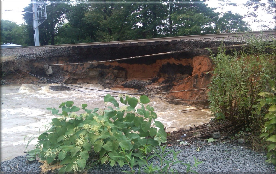
North Jersey Coast Line-track bed undermined as a result of Hurricane Irene
