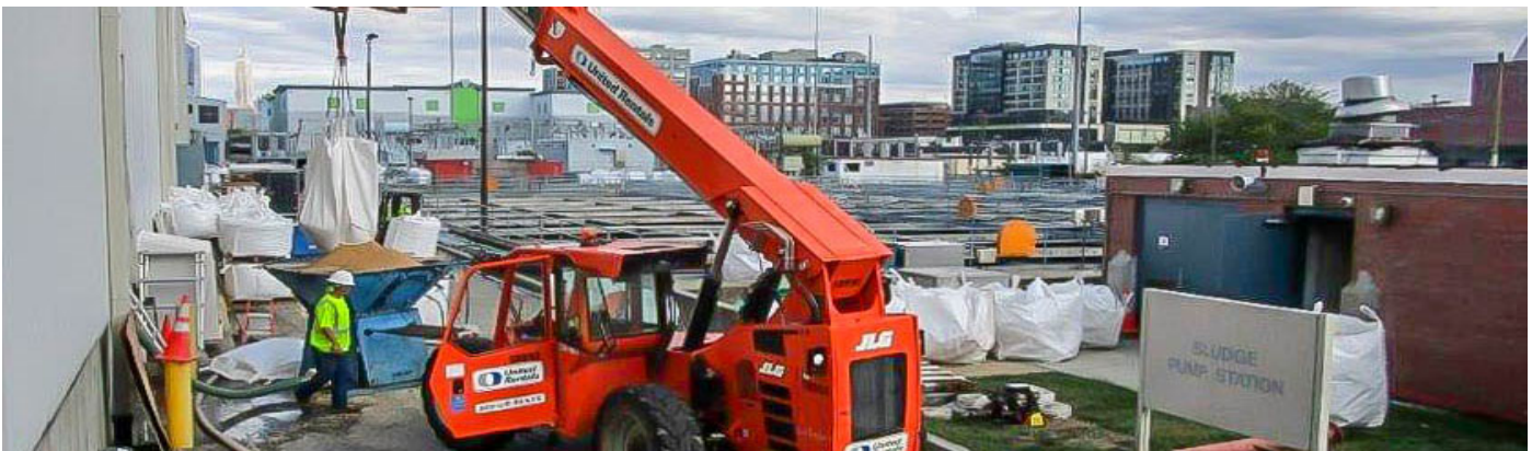
North Hudson SA WWTP Improvements, Purac, Phase 3 Physical System Improvements. SFY2022 Loan: $16,755,831
