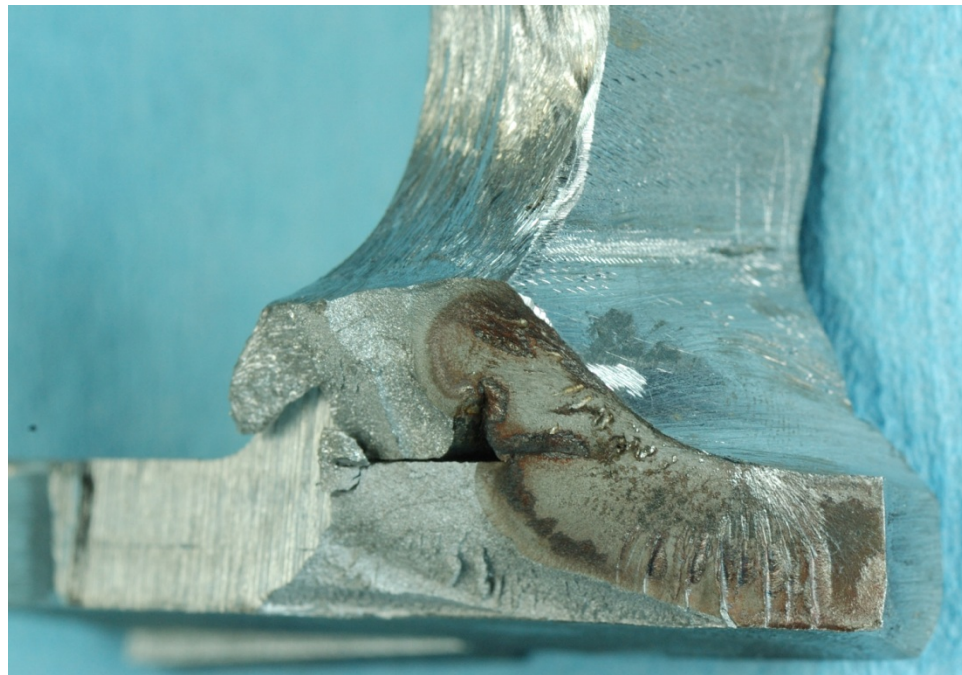
Figure 224. View of fracture surface to the south at about 35 degrees from the rib soffit in MU3 showing the deviation of fracture plane through the weld
