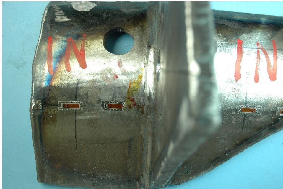
Figure 204. Portion of rib and floor beam containing the north side crack cut out of the mock-up specimen MU1
